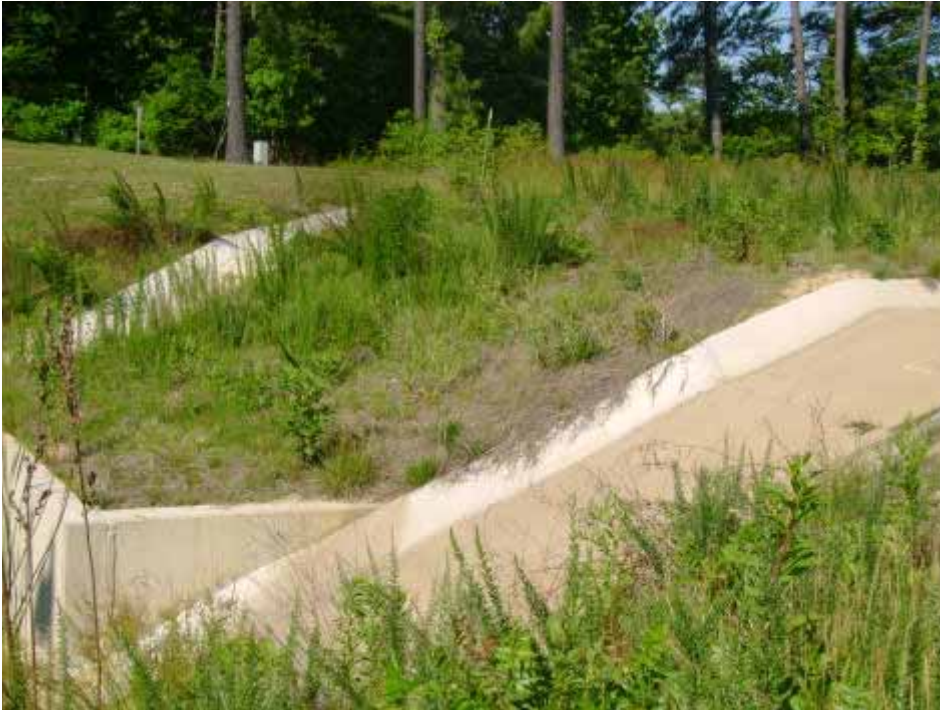
Photo #3: Concrete flumes into rip-rap lined basin at the southeast corner of the site. Note the poor permanent stabilization of the embankment.
