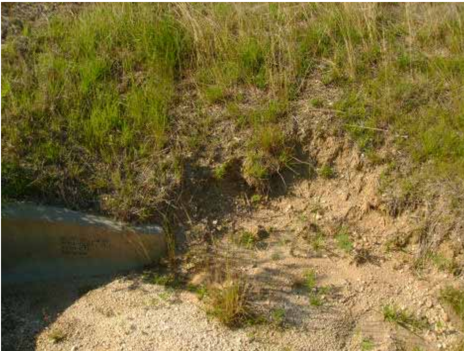
Photo #2: Note the erosion of grass channel embankment at upstream end of culvert.
