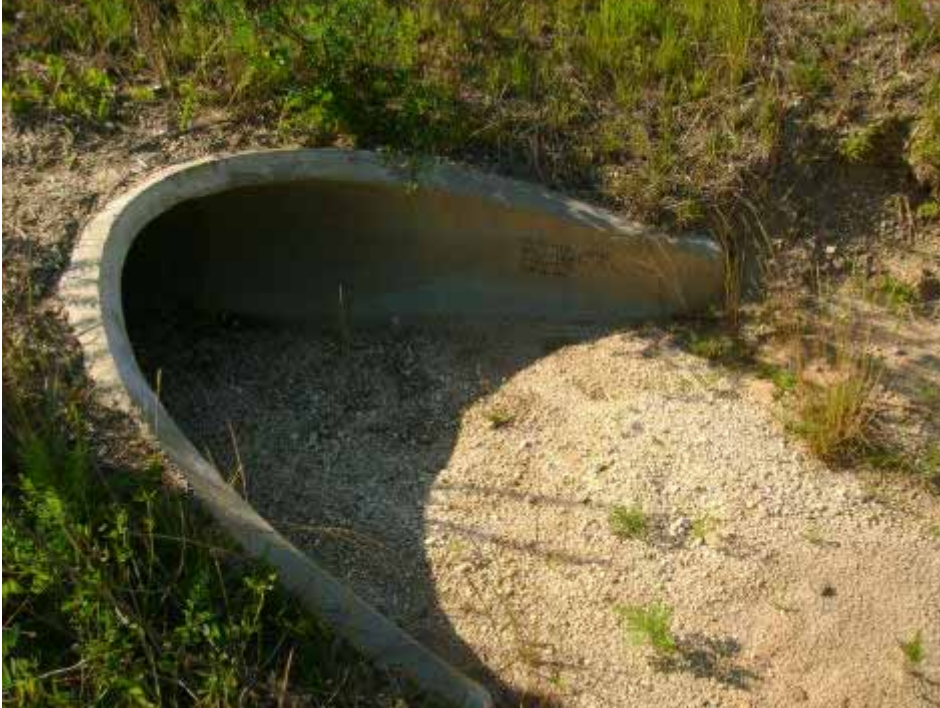
Photo #1: Buildup of sediment was noted within the grassed lined channels. This photo shows the sediment that has accumulated within the culvert beneath access road to site.
