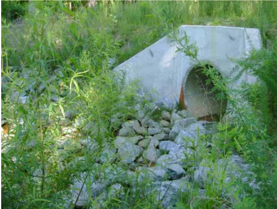
Photo #7: Image of endwall at outfall into the 100 Year Floodplain of Pine Hill Run. Note the sediment laden runoff within the storm sewer.
