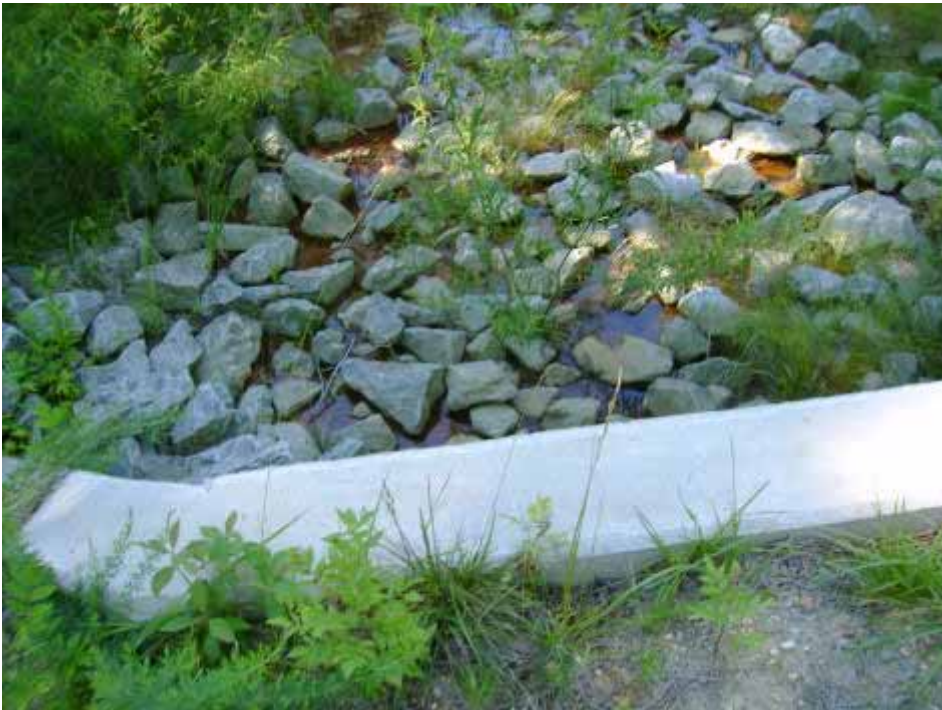
Photo #6: Rip-rap lined outlet protection at endwall of outlet pipe. Note the presence of sediment laden water within the rip-rap lining.
